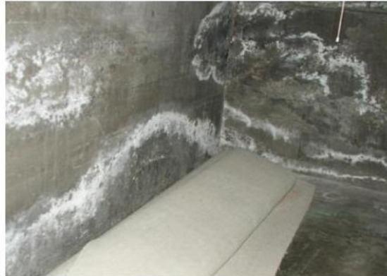
Efflorescence on plaster
