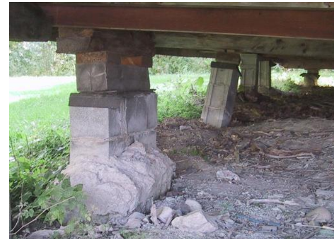
Figure: Foundation Heaving https://woodgears.ca/cottage/foundation.html
