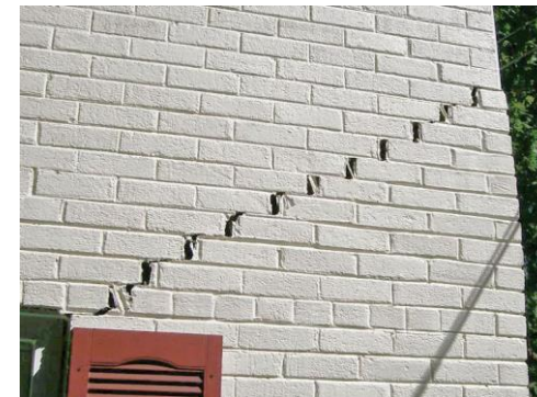
Figure: Crack on the building
