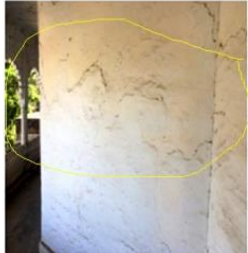
Figure 2: Wall of Labour Court Type- Medium (Non-Structural Crack)
