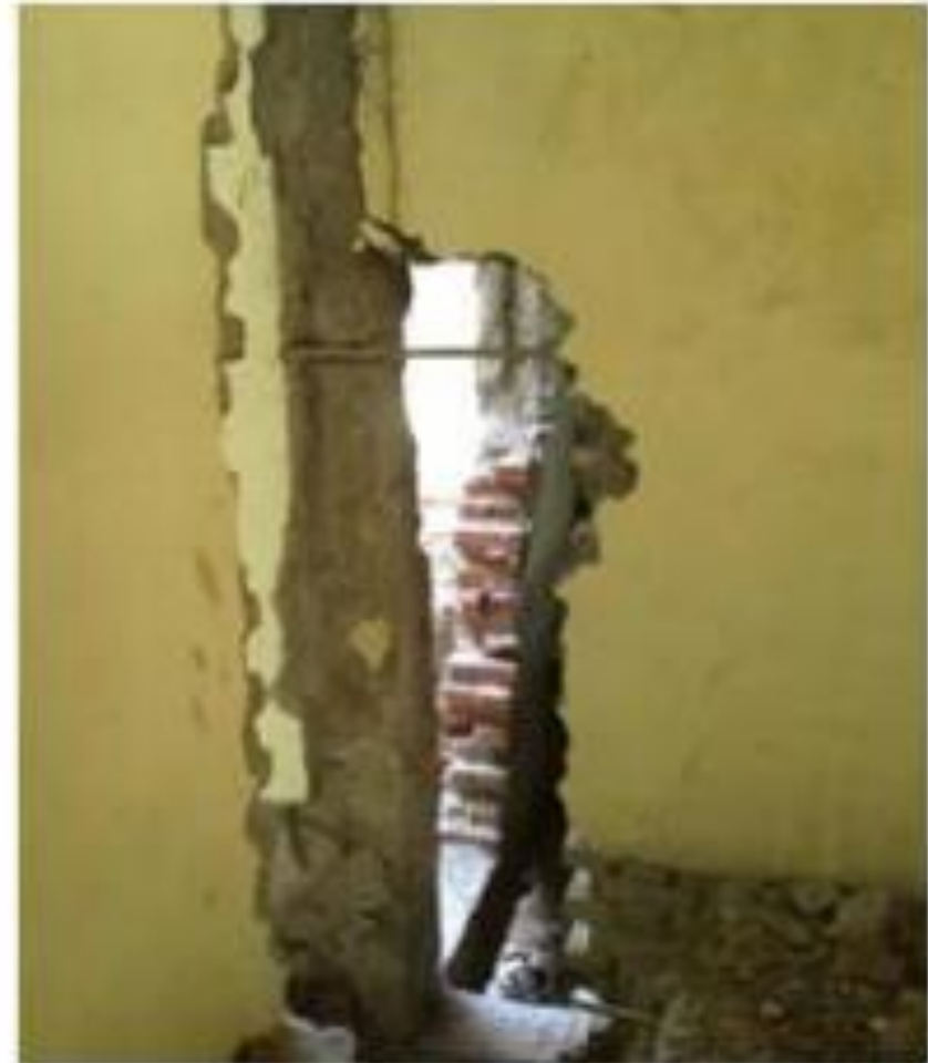
Figure 4: Rear Column Type- Major Structural Crack Cause- Settlement of Foundation
