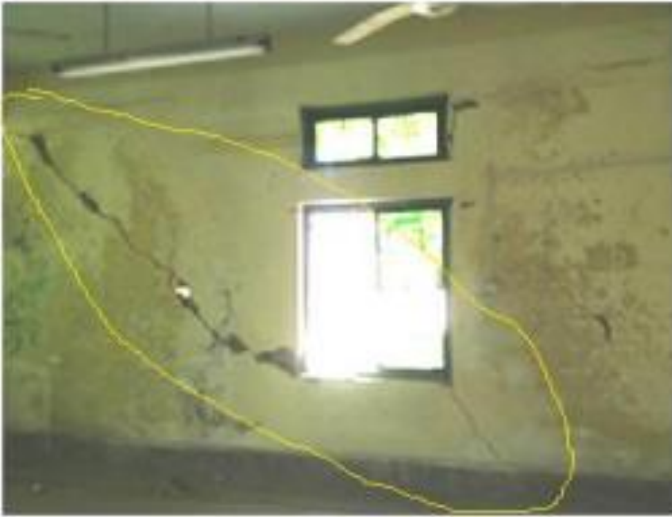
Figure 3: Long Wall of Sir Alexander Cunningham hall (political block) Width – above 2mm Type- Wide, non-structural crack Shape- Stair Step Crack Cause- Settlement of Foundation
