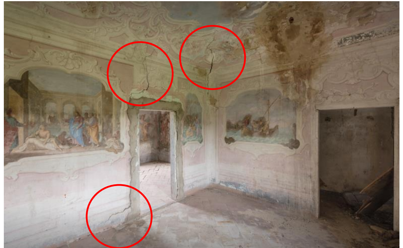
Figure :Cracks (Source: Stouhi,D.( 2019,March 30):Online) https://www.archdaily.com/913780/dust-cracked-walls-and-enchancing-artwork?ad_medium=gallery
