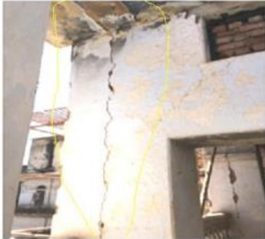
Figure 1: Column at industrial court Type- Major Structure Crack Shape- Vertical Crack Cause- Thermal variation, due to joint
