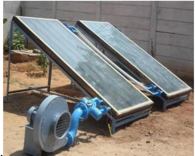
Solar air heater
