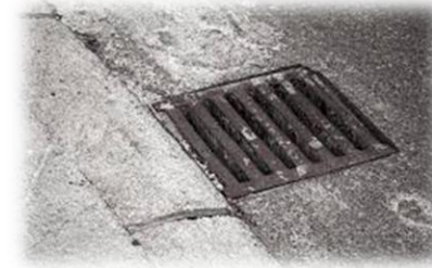
Figure 10: Surface water drain (©sunil Rakhal, 2021)
