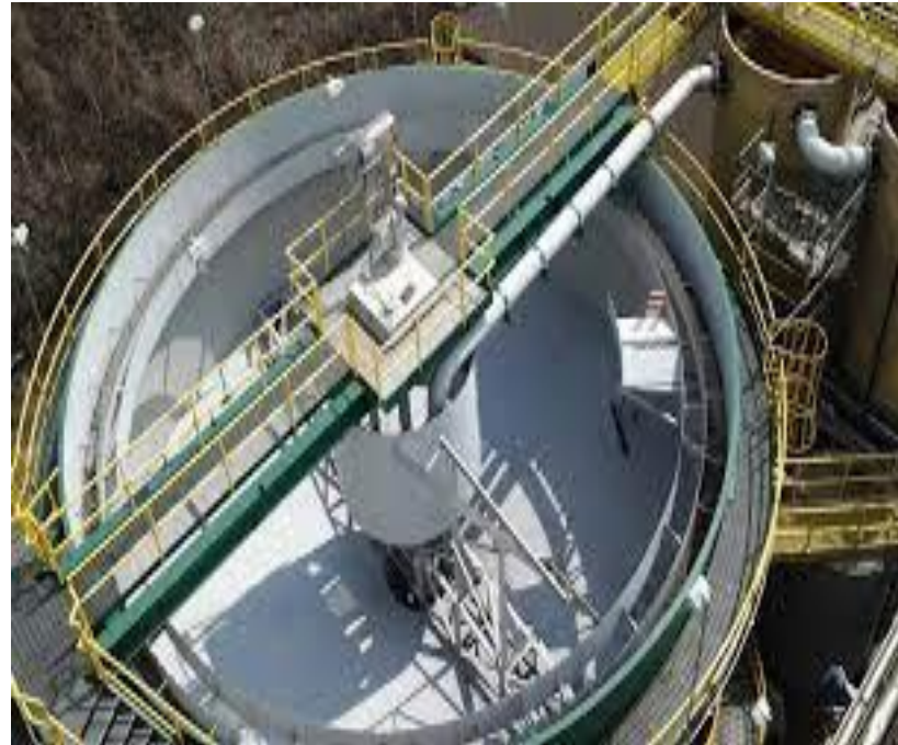
Figure 5: Clarifier source: (www.monroeenvironmental.com/water-and-wastewater-treatment/circular-clarifiers-and-thickeners/, n.d.)
