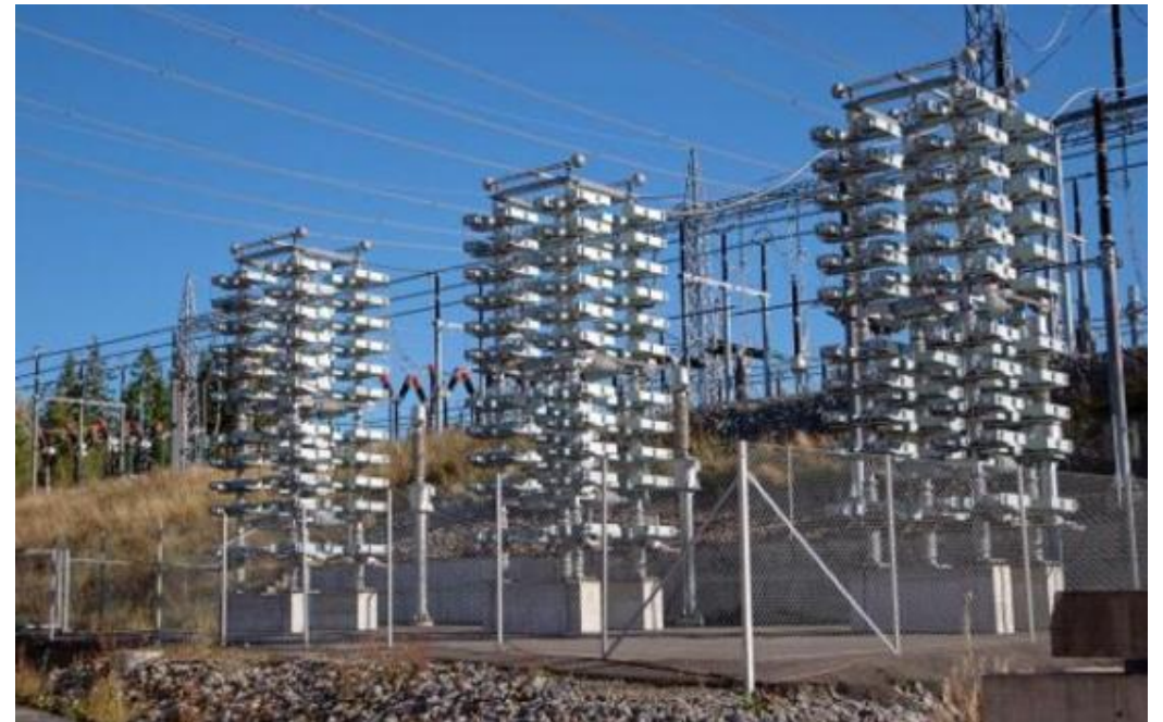
Figure 4: An ABB Shunt Capacitor Bank [3].
