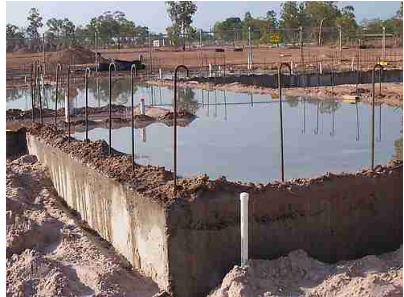
Bradley, Bill (2025). A concrete slab ponded while curing [Photograph] . Wikimedia Commons. https://commons.wikimedia.org/wiki/File:Curing-concrete.jpg
