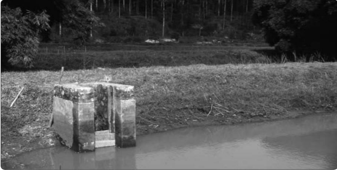
Figure 2.2-8. Although more expensive to construct, monks are sometimes used instead of standpipes. In this example, some of the upper boards have been removed to lower the water level in the pond.
